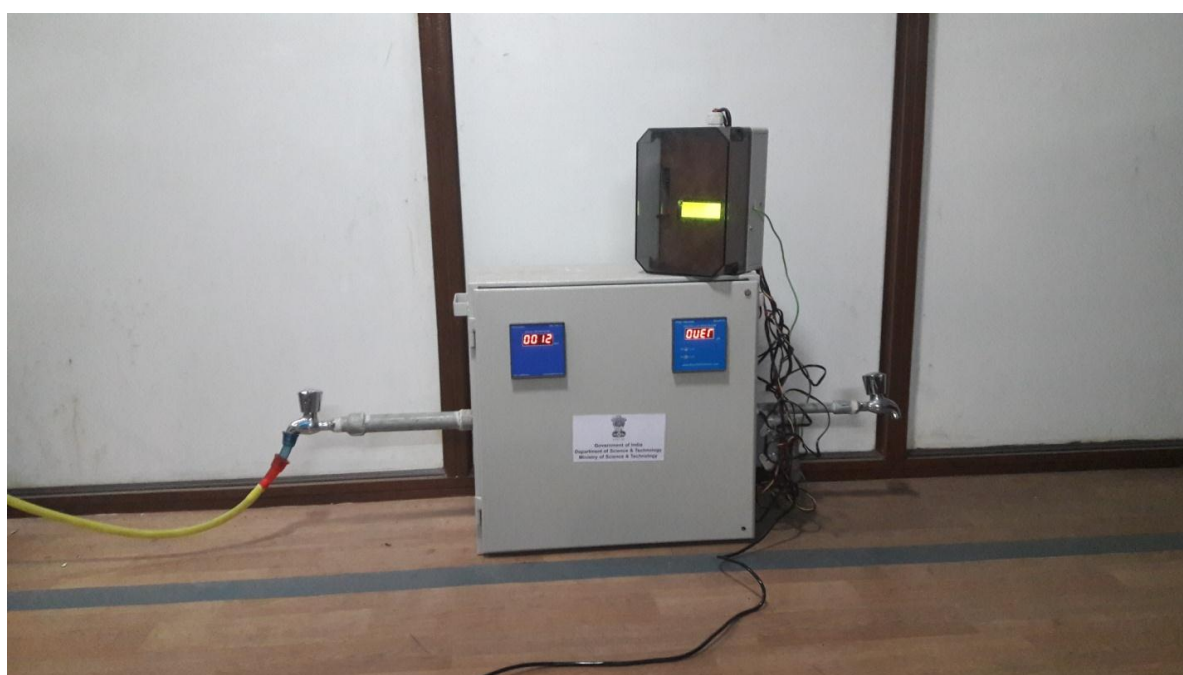
The smart water quality monitoring system, developed at the WSN and IoT Laboratory of the Department of Information Technology
